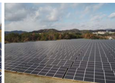
Ichigo Higashi-Hiroshima Saijocho ECO Power Plant
