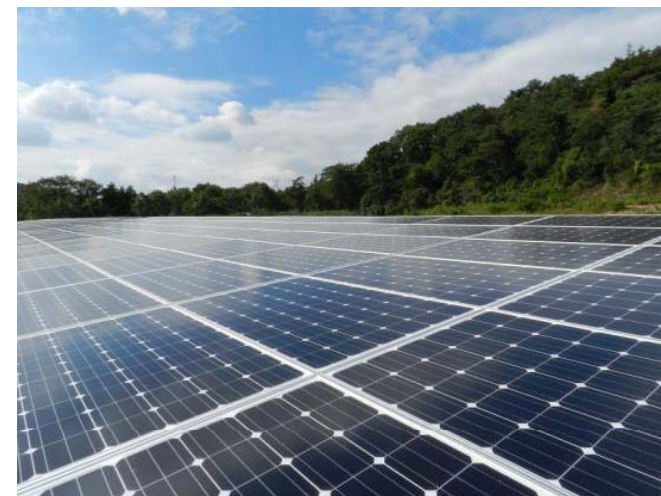
Ichigo Kiryu Okusawa ECO Power Plant (Online Sep 2013)
