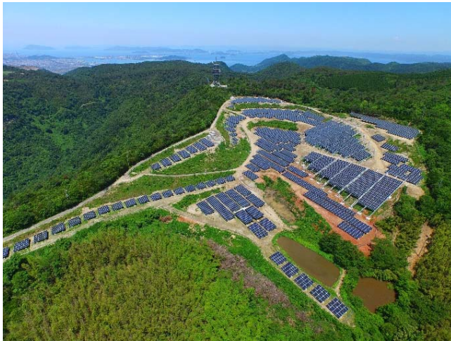
Ichigo Takamatsu Kokubunjicho Nii ECO Power Plant (2.43MW)
