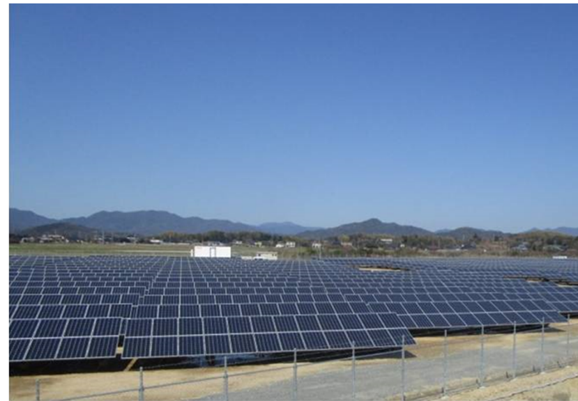
Ichigo Yamaguchi Sayama ECO Power Plant
